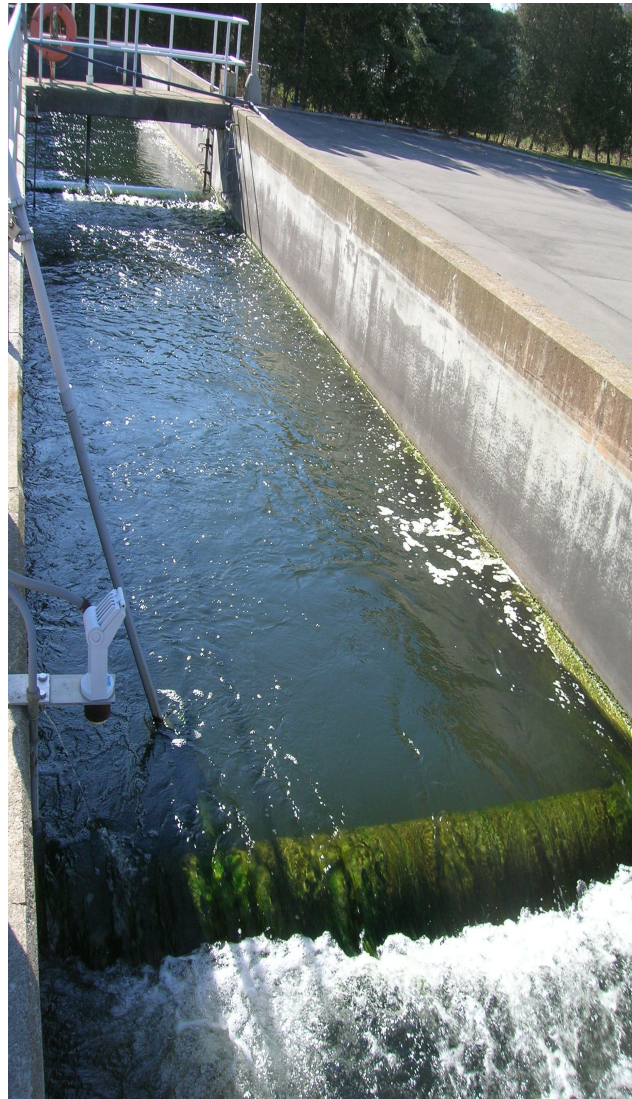
Secondary clarifier photo 5: Aeration at the end of the secondary clarifier
