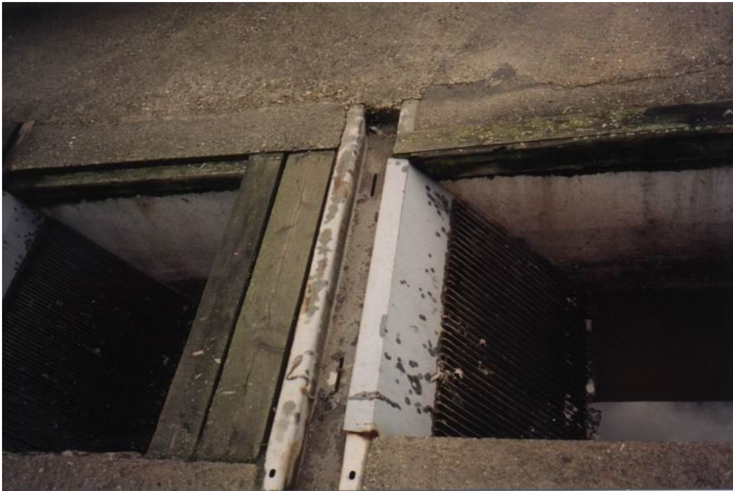
Bar screen: This screen removes large objects to protect the machinery in the plant (image not from Cortland)
