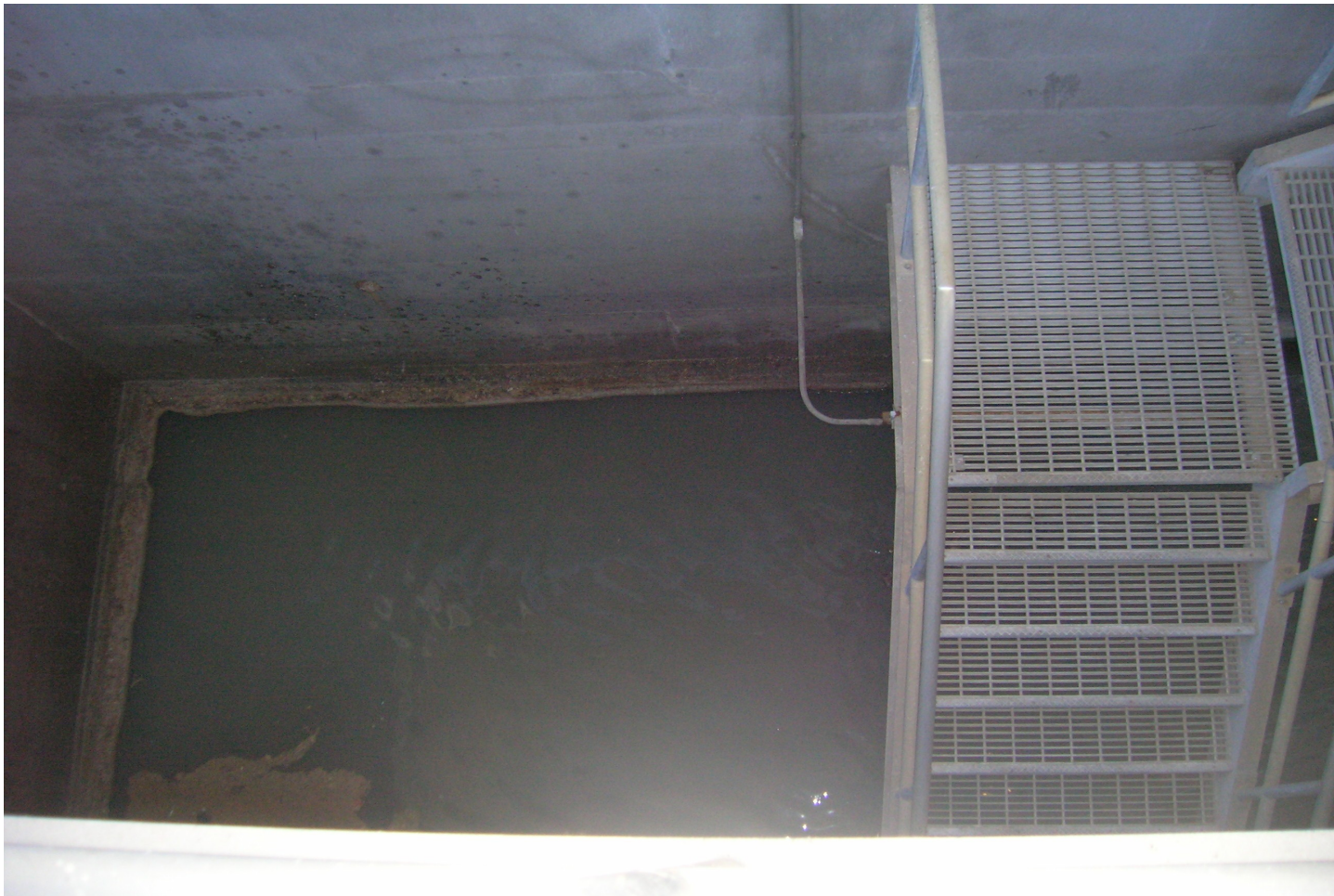
Raw sewage influent well: Raw sewage is collected here with waste sludge (excess bacteria) from the secondary clarifier.
